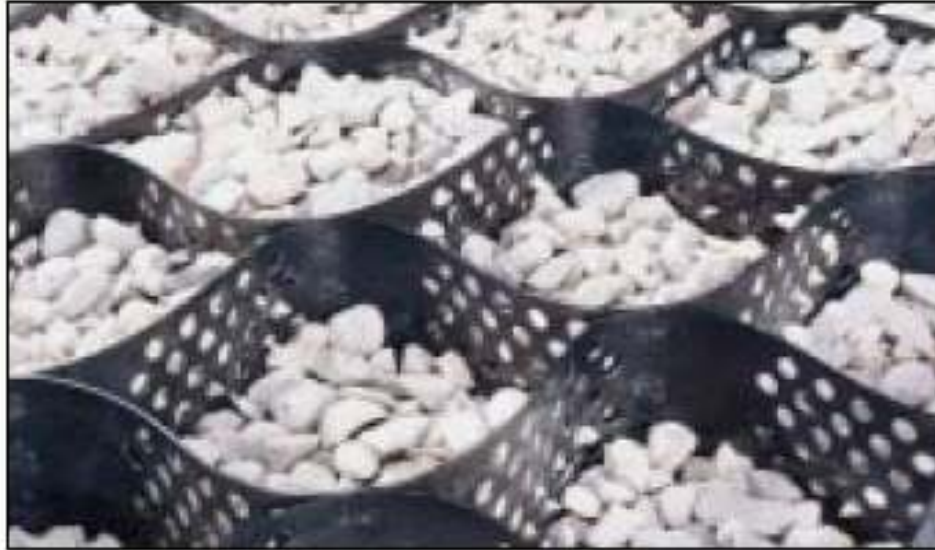
Confined Cellular System (CCS) – gravel filled Soil will be placed on top of gravel
