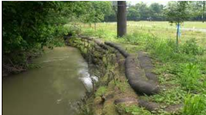
Erosion control tubes (Filtrexx photo)
