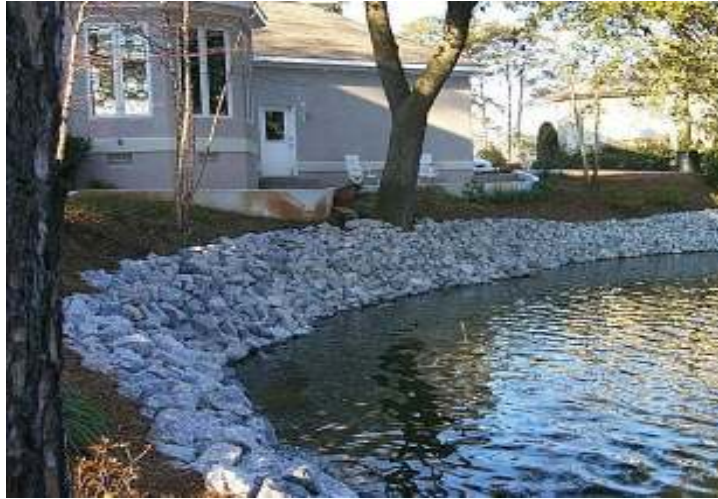
Riprap. Photo shows riprap above water line. Riprap above the waterline at Bo-Rit will be soil-choked and planted.
