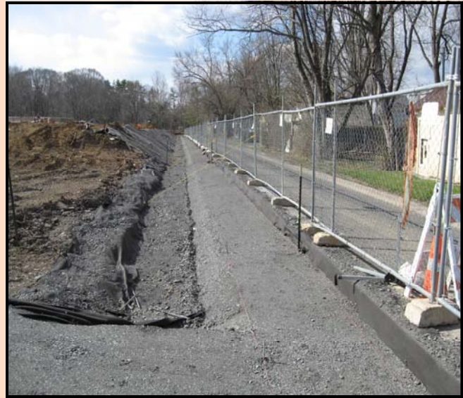
View of the working area along the alleyway by the Rose Valley headwall, facing north.
