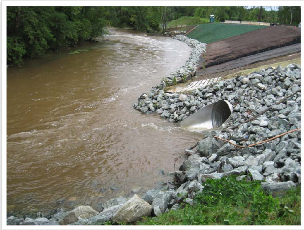
Confluence of Tannery Run and the Wissahickon Creek & view of the Phase V Slope
