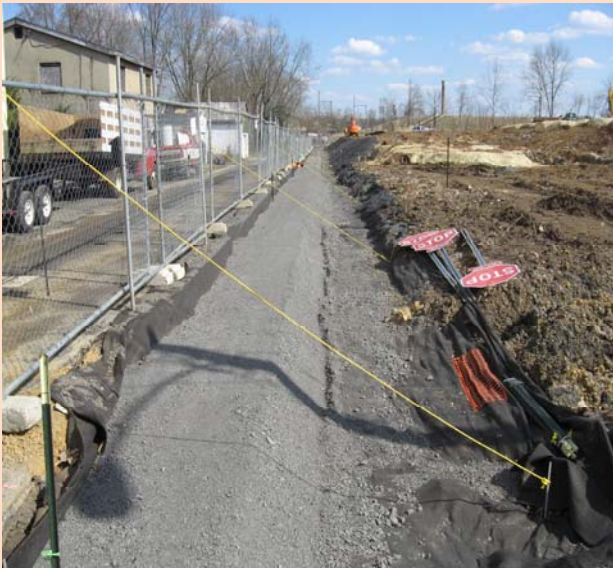
View of working excavation along the alleyway at the north end of the Site, facing south.
